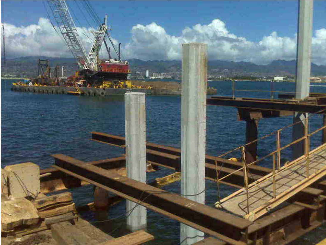
Figure 2.1 Navy Magnetic Silencing Facility shown during construction in Pearl Harbor using 24” octagonal piles prestressed with 26 - ½”, 240 ksi austenitic stainless steel strands (Courtesy Foundation & Geotechnical Engineering, Plant City, FL).
