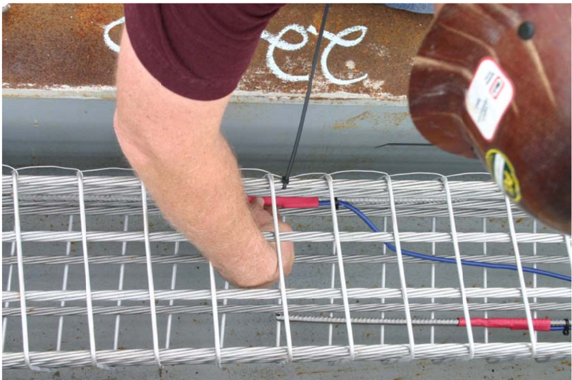
Figure 5.12 Embedded sister bar gages installed at mid height, 28 in from each end.
