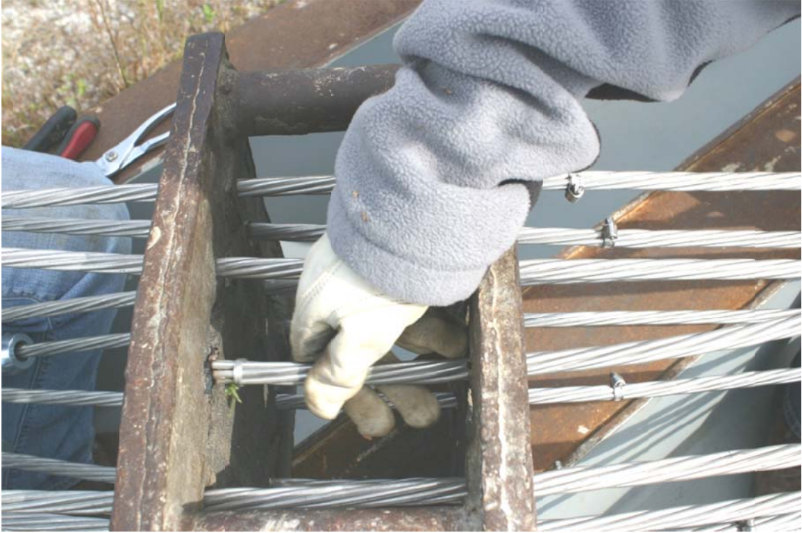
Figure 5.6 Each strand threaded through the appropriate hole in the pile header blocks.
