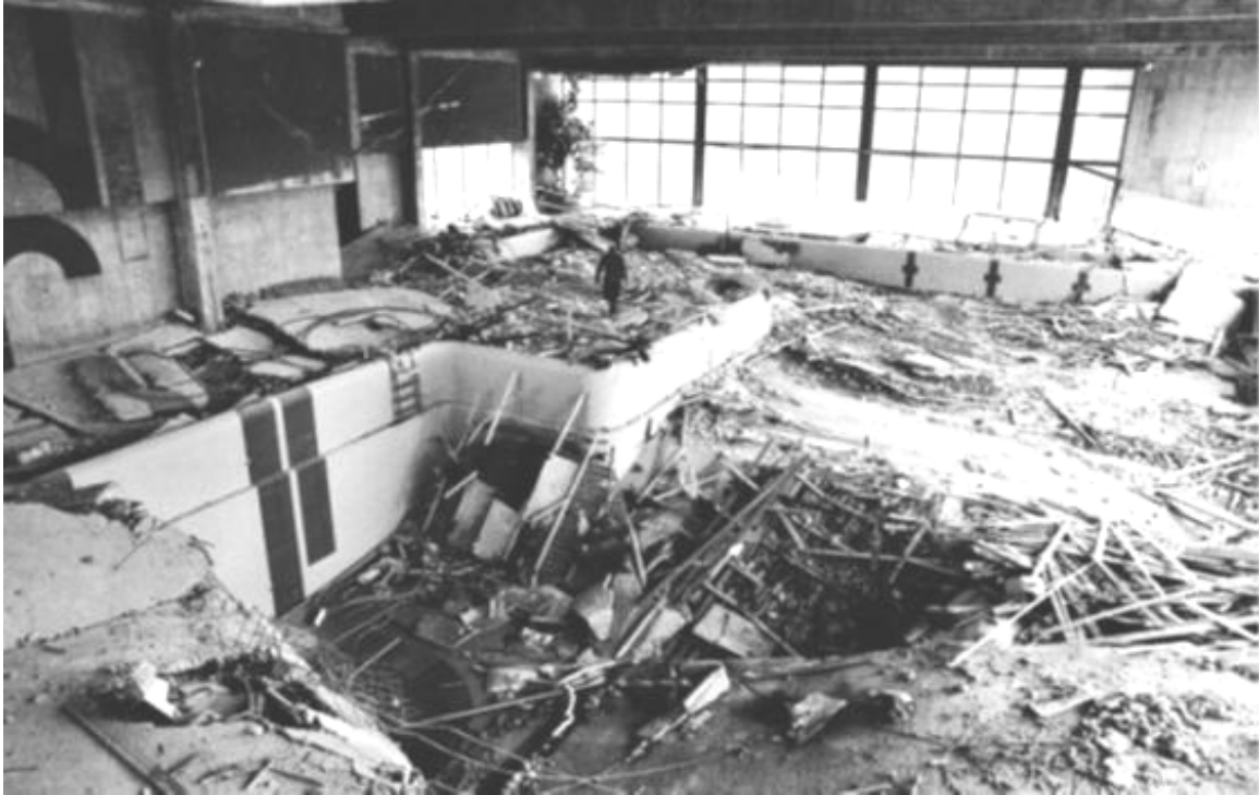
Figure 2.4 Suspended ceiling collapse of Uster swimming pool caused by transcrystalline stress corrosion cracking (Faller, 2003).
