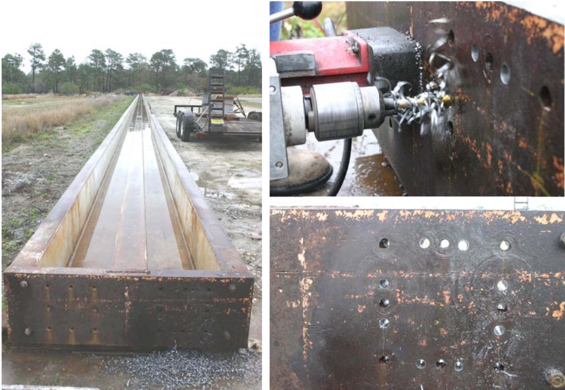
Figure 5.1 400ft prestressing bed (left); drilling modification to header plates (top right); 12 strand pattern superimposed on 8 strand header plate (bottom right).
