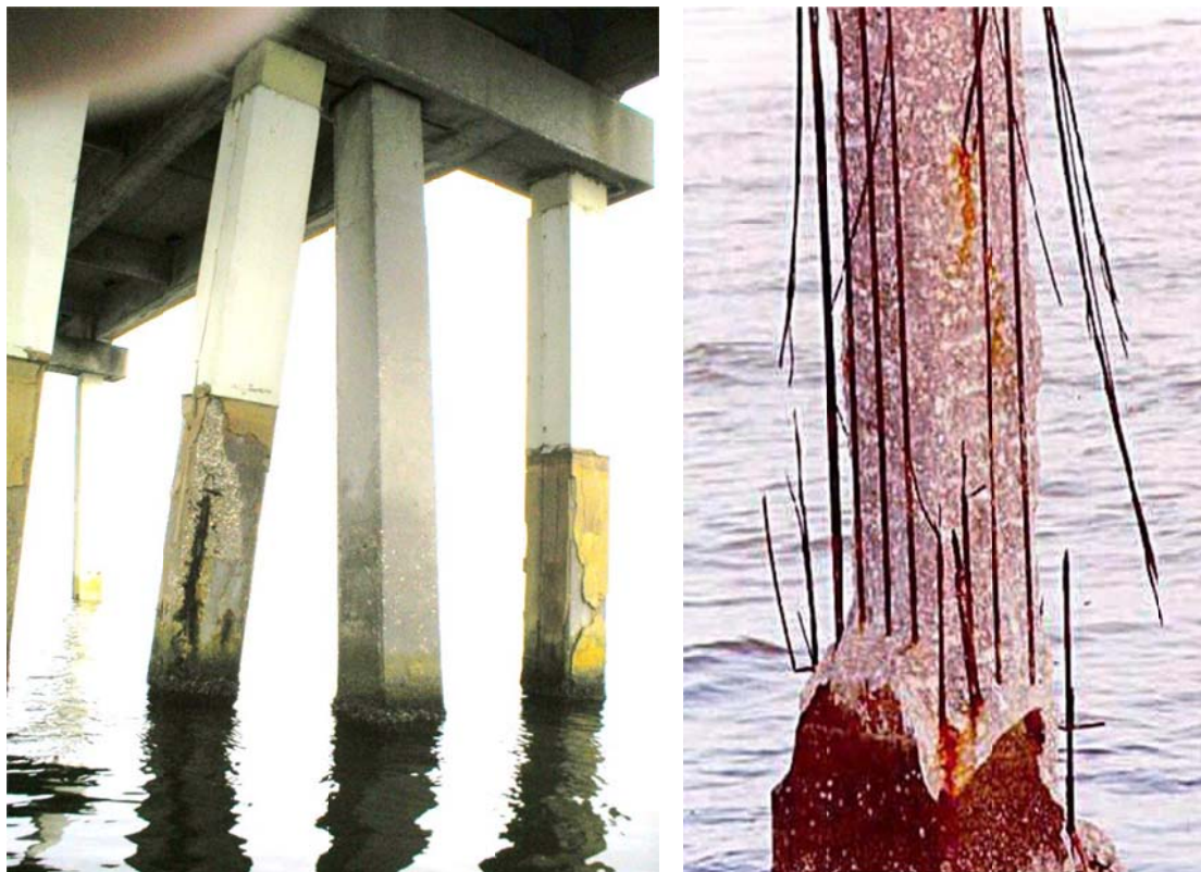
Figure 1.1 Pile damage caused by corrosion.
